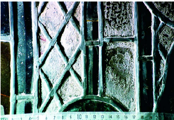
Figure 2: Detail of a stained glass panel from the Dome in Altenberg, Germany; the density of the corrosion crust depends on the composition of the glass and thus varies with in one panel (photograph provided by the Dombauhütte Köln, Germany)
