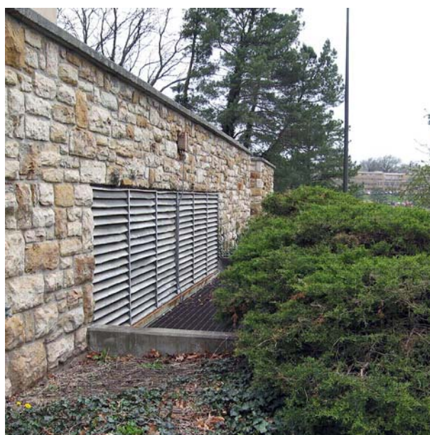
Figure 6: Image showing fresh air intake grill located very near vegetation and damp soil.
